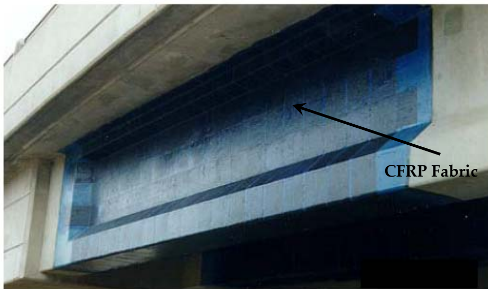
Fig. (2-6): Shear Strengthening of a Reinforced Concrete Bridge Girder Using CFRP Sheets, [ISIS-EC-2, 2006].
